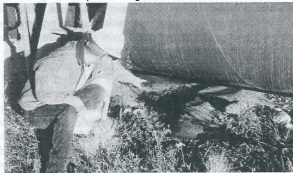
Figure 4 Run-off entry point that led to erosion.
